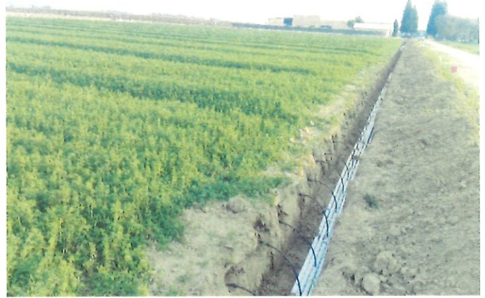
Figure 2 Connecting sub-surface drip lines with water supply at Kearney. There were 6 lines to irrigate different sections.
